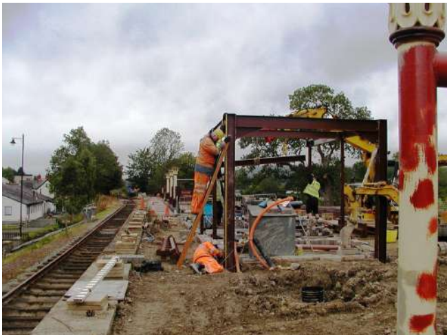
Frame under construction Ron Stansbie and John Mason Checking measurements Photo: PR
