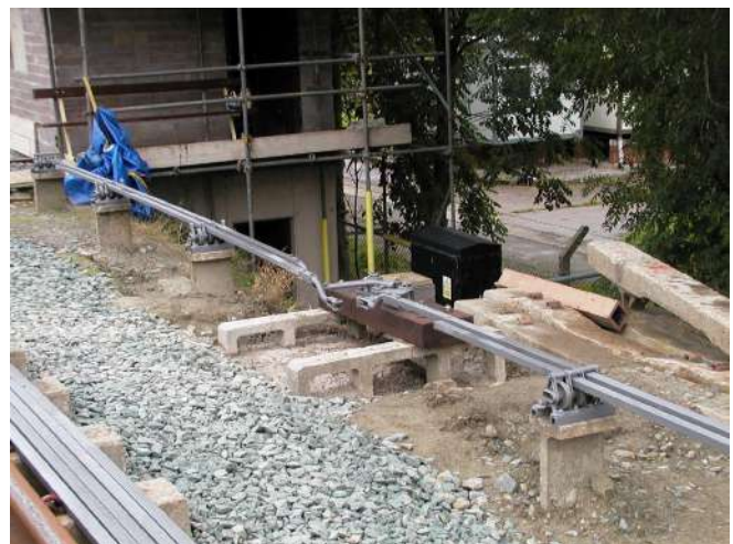
Point rods and crank near the signal box base Photo: PR
