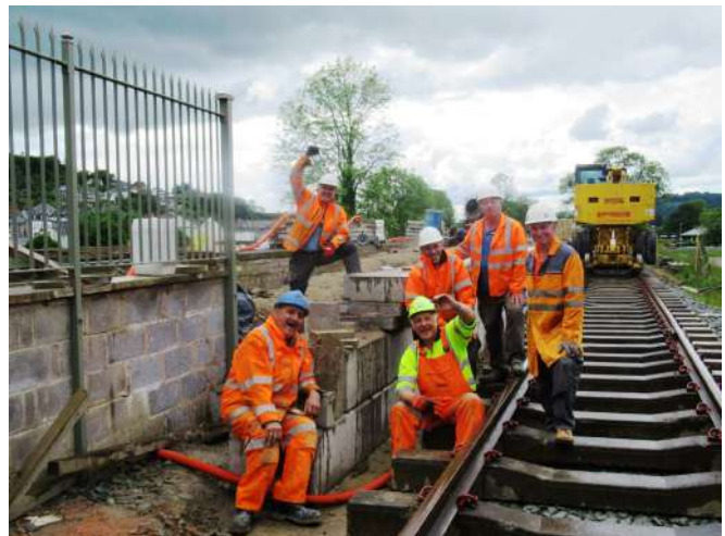
Gang led by John Mason complete the block work on the east end Photo: GJ
