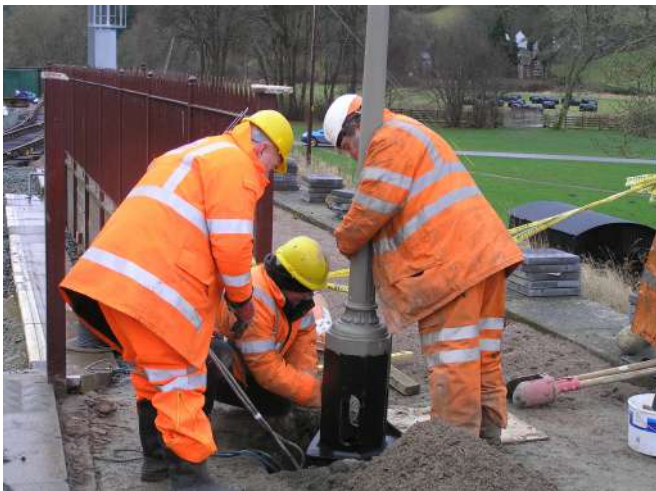
Site electrician Phil Coles cabling up a lamp post at the east end Photo : PR
